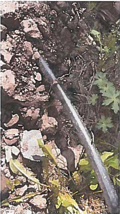
Photograph 8: Exposed water line on Balsam
